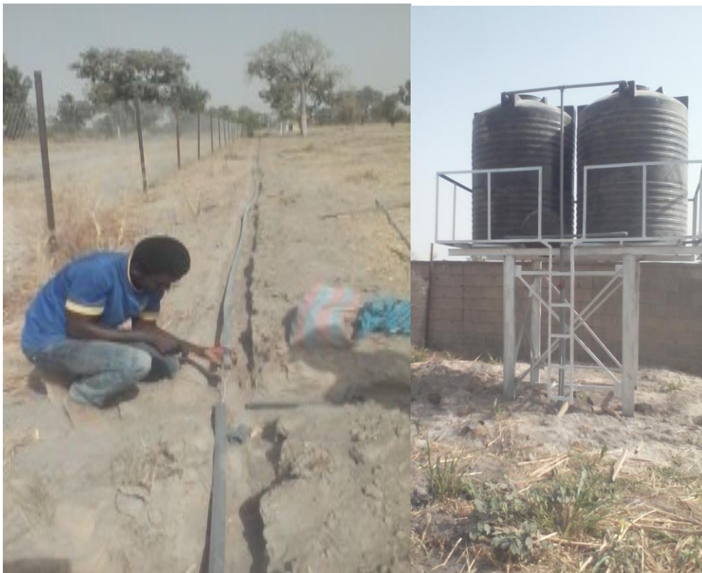
Fig. 8. The pipes layout for the drip irrigation system and overhead tank in the research area.
